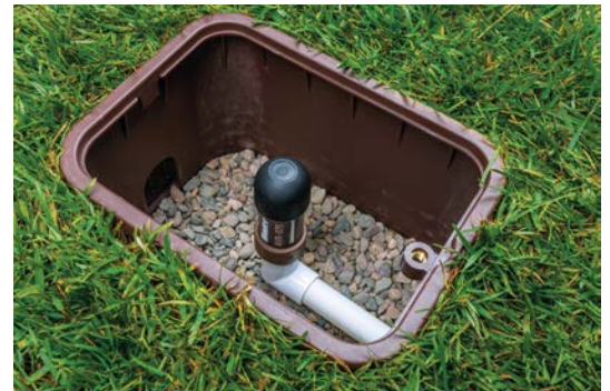
Air/Vacuum Relief Valve Installed
