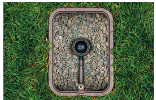
Automatic Flush Valve Installed
