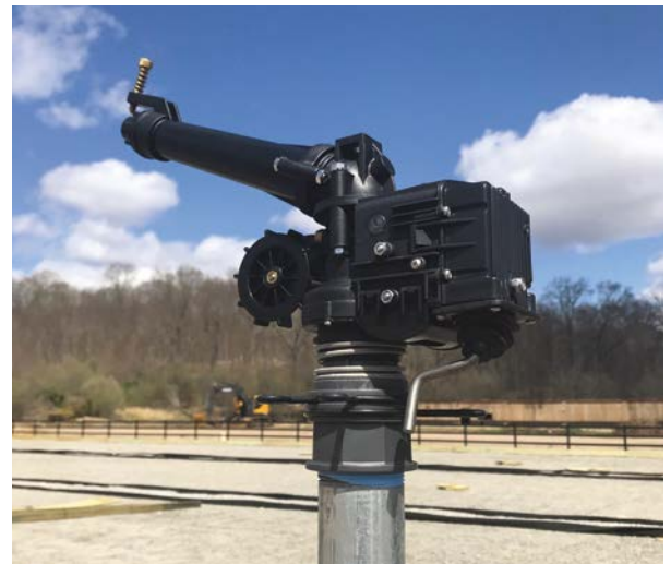
ST-1200-BR Rotor Installed
